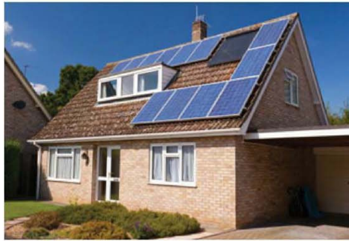
Solar panels on the roof help provide heat and electricity.
