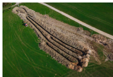
ground source heating
